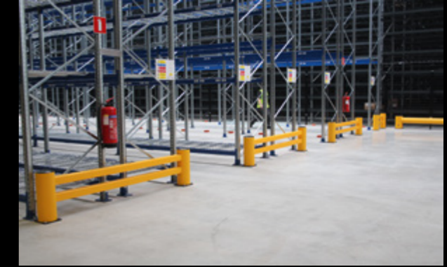
▶ Rack End / rack protection
